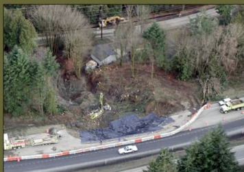
Figure 4. Slide on Highway 101 near Road 8.
